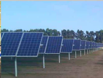
Solar Array for SunPower at Oxnard High School
